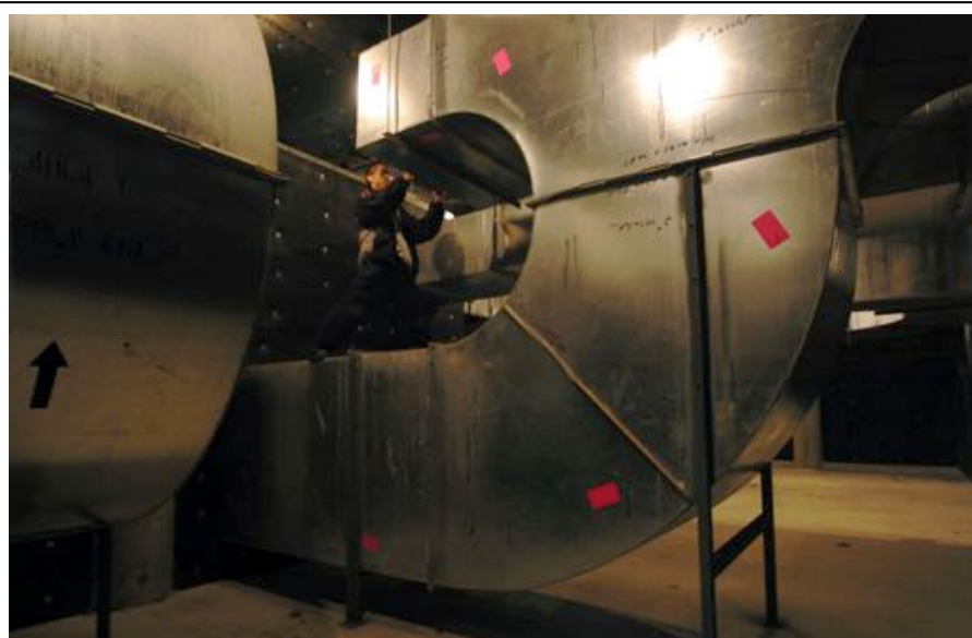
Figure 2. Kiyoshi Kuroiwa performing acoustic measurements in the plenum underneath Hammerson Hall at the Mississauga Living Arts Centre. Mr. Kuroiwa is holding a sound level meter but it is blocked from this view by the duct.
